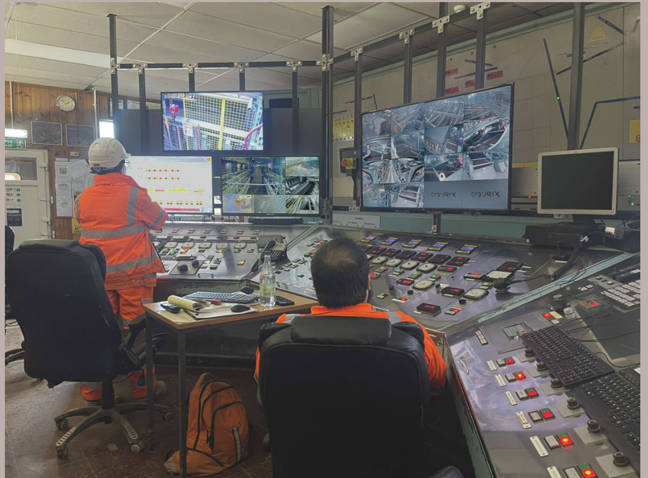
Site control room showing live feeds from Ciqurix video detectors.
